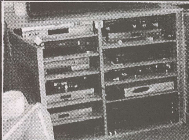
Carman's "DX Earth Station" is loaded with gear that remains hidden when cabinet doors close.
