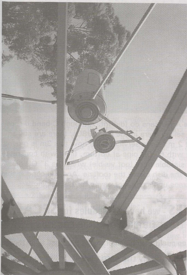
ONE method to hang second LNB + feed offset from prime focus to receive additional offset satellite without moving dish.
