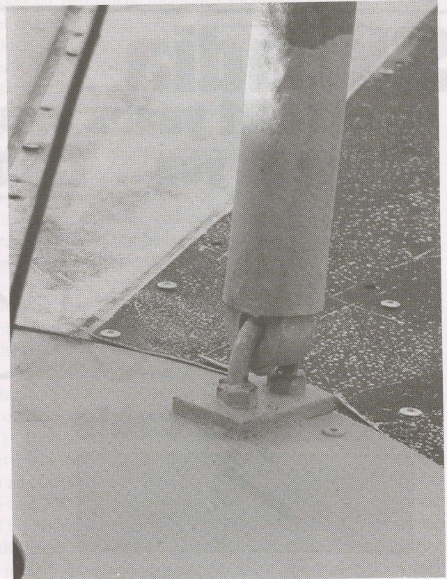
Feed support pipe has universal joint at base with two supports to perimeter of the dish; one N-S, the other E-W. This has many advantages over a standard tripod mount.
