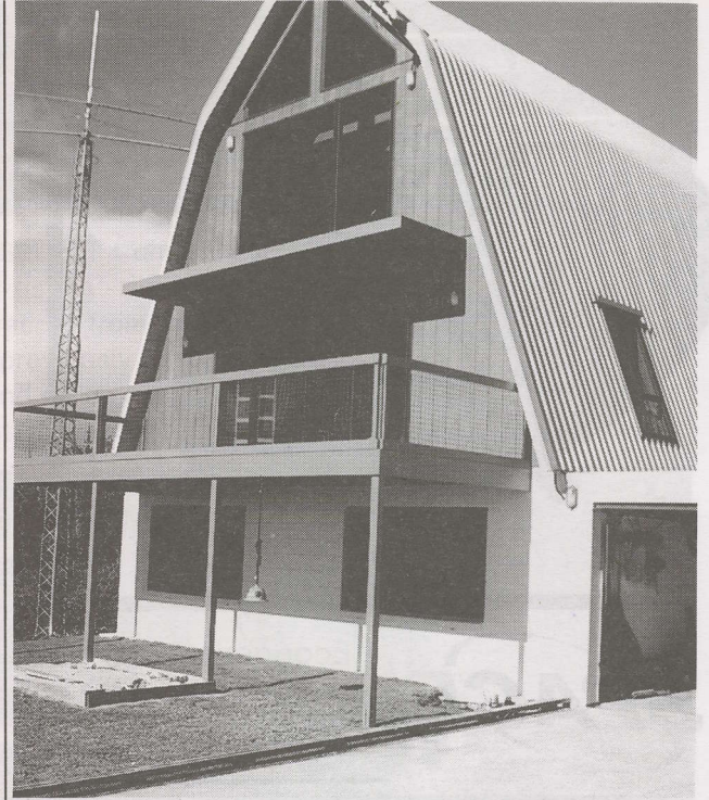
INSIDE the glass window, second deck (third floor) above ground is discone antenna, 10-watt L-band transmitter. Note corrugated steel roofing (see text).
