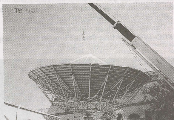
Lifting the beast in Illinois - it became known as "Mullane's White Elephant."
