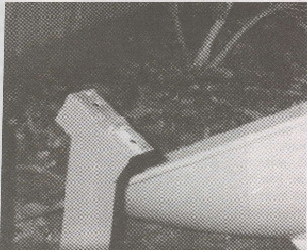
Weight of dish, 'loaded' with wind, pulled mounting brackets out of brick veneer wall which was in danger of collapsing if the dish was not removed.
