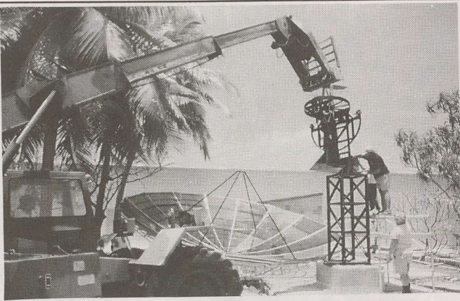
Bob Maddock guides the mount to the working position atop the tower.
