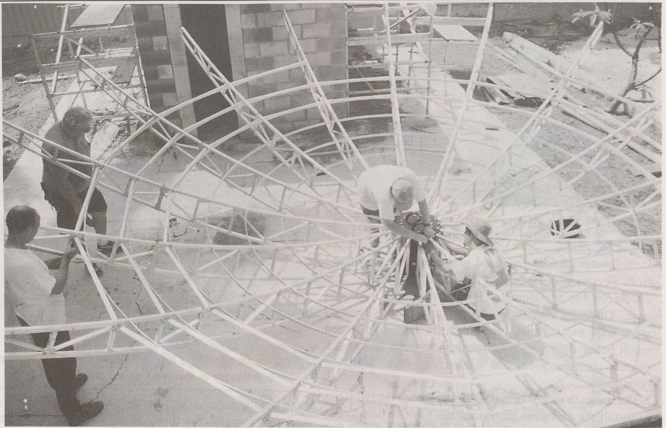
The dish is really starting to take shape. Bill Kostka and Jim Bramblett tighten the truss bolts at the spool while Robert Ferguson and George Lord install the last of the mesh support brackets.
