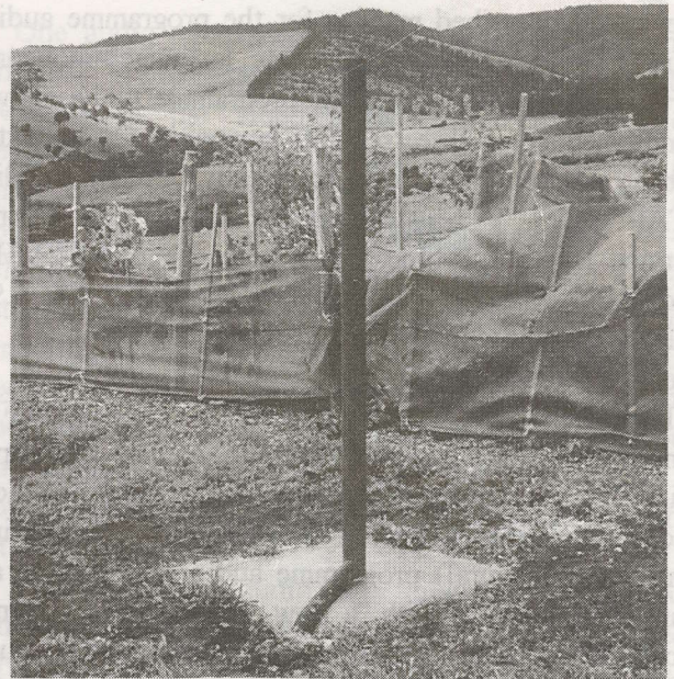
Schedule 80 pipe is placed in hole and concreted in place; pole should be vertical with respect to ground, checked two times; once on each "side."
