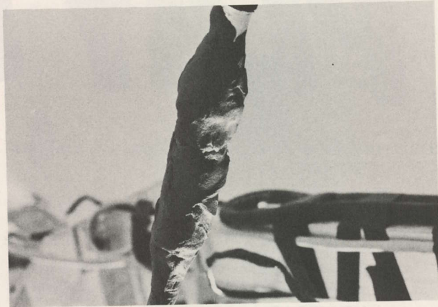
COAX SEAL applied — it feels like damp putty and molds and conforms to the fitting being 'wrapped.'
