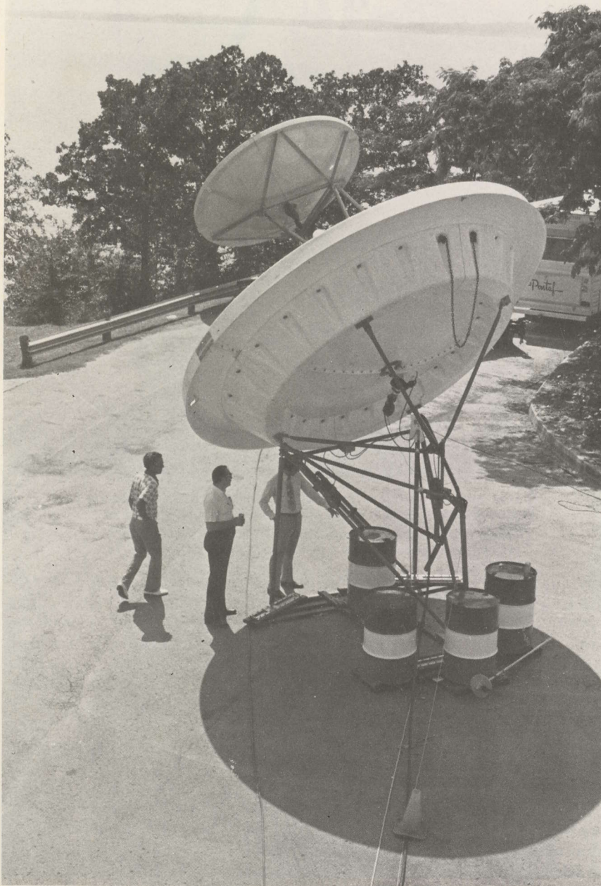
BIG AND LITTLE OF IT — Actually both terminals are about the same (4.5 meter) size. The closer terminal is the Prodelin fiberglass structure on its show mount. Behind it, on a trailer mount, is the Andrew solid metal terminal. Both looked South/southwest over Fort Gibson Lake.
